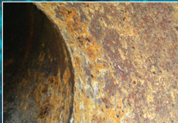
Pitting corrosion around exhaust discharge.
