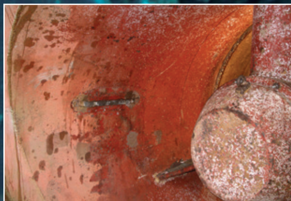
Corrosion around bow thruster.
