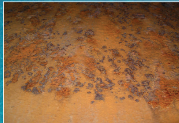
General corrosion on hull plate.
